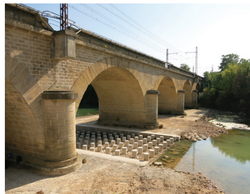
Riprap fishway at sill level under the Vidoule Bridge in Gallargues le Montueux
