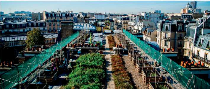
Experimental vegetable garden rooftop at AgroParisTech using urban waste as technosol components © Baptiste Gard/Vinci
